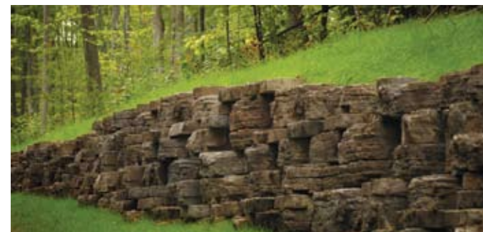
Grade slope to rise above top blocks, giving the look of natural outcropping in the bank. (Design must account for surcharge loading)
